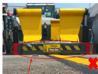
Cradle not fully lifted
